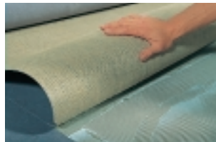
Folding back the trimmed sheets, either half-way back in the case of rooms or lengthways in the case of corridors etc...
