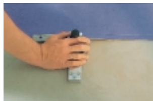
Cutting the first edge of the sheet is best done with a linoleum edge cutter or strip trimmer.
