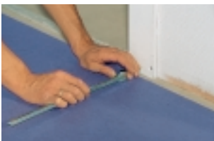
Transferring the shape of a doorpost to the linoleum with the help of a bevel.
