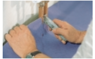
The loosely-laid sheets are cut in, around a radiator in this case.
