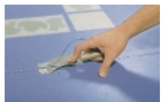
The weld rod is trimmed in two operations, first with the trimming guide fitted, then with the bare blade.
