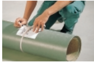
The sheets are cut to size, marked, loosely re-rolled and placed upright to acclimatize to conditions in the room.
